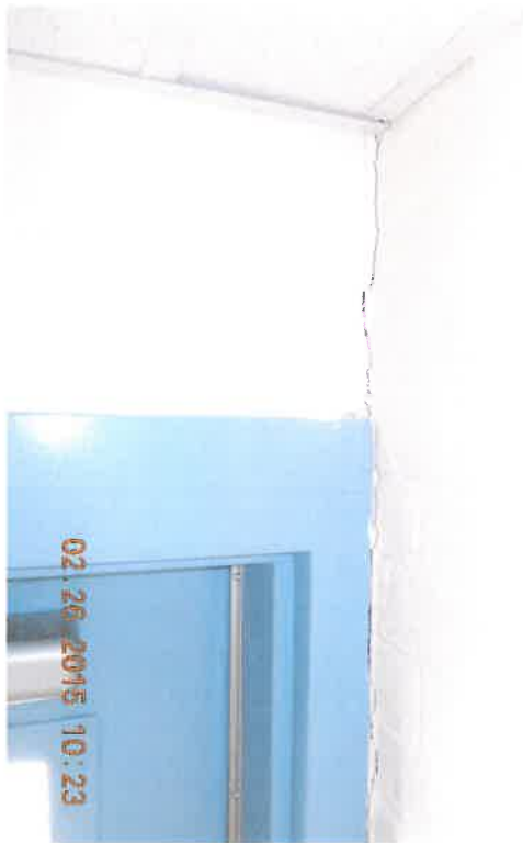
Natural shrinkage. New wall meets old.
