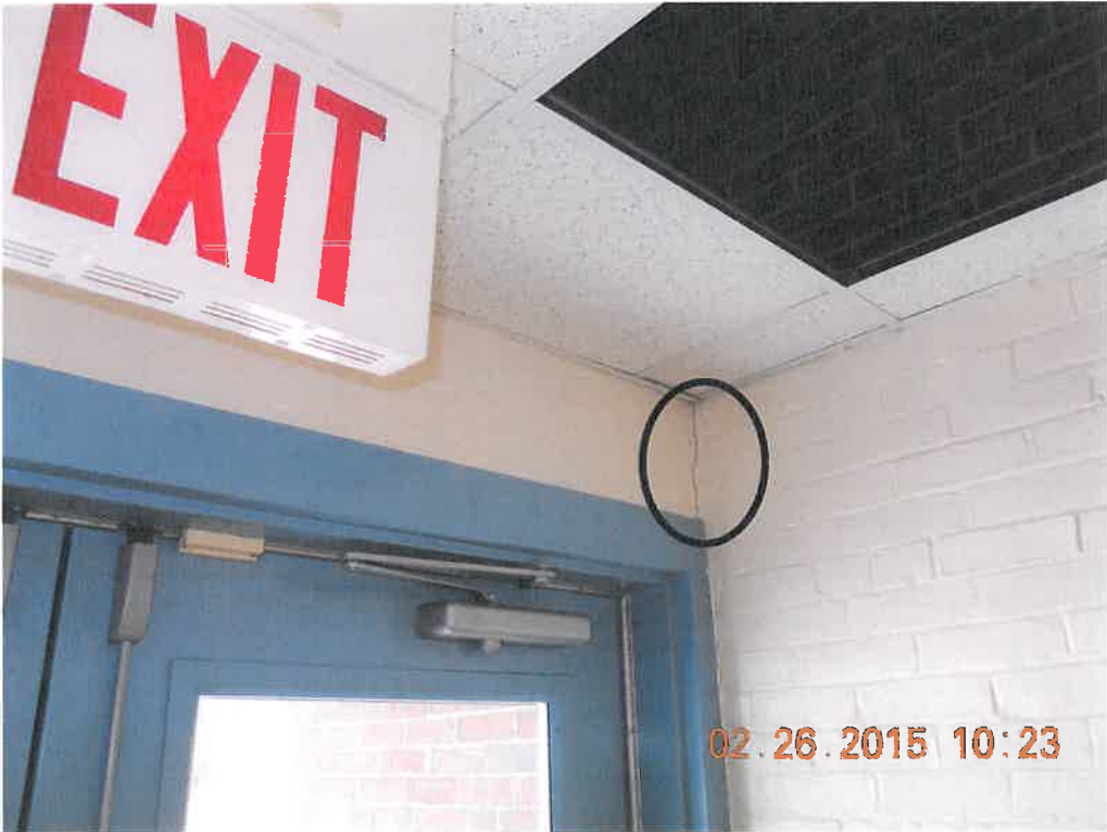
Corridor wall crack at exit door
