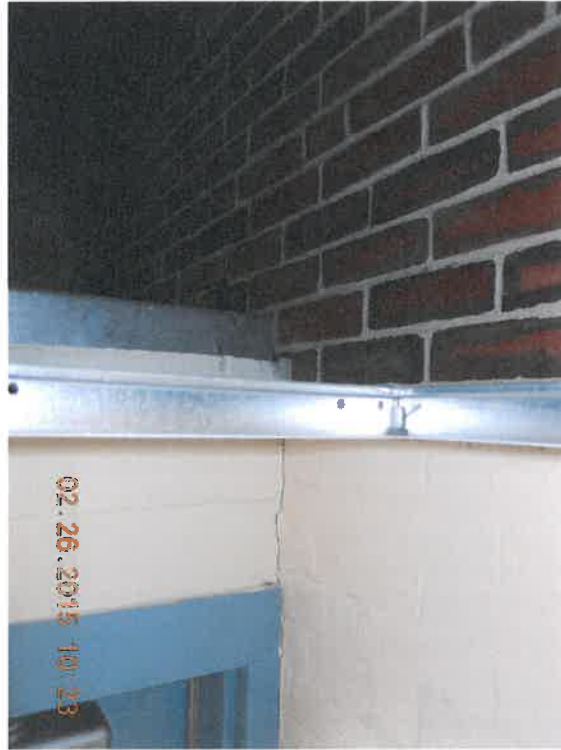
Corridor wall crack at exit door and above ceiling
