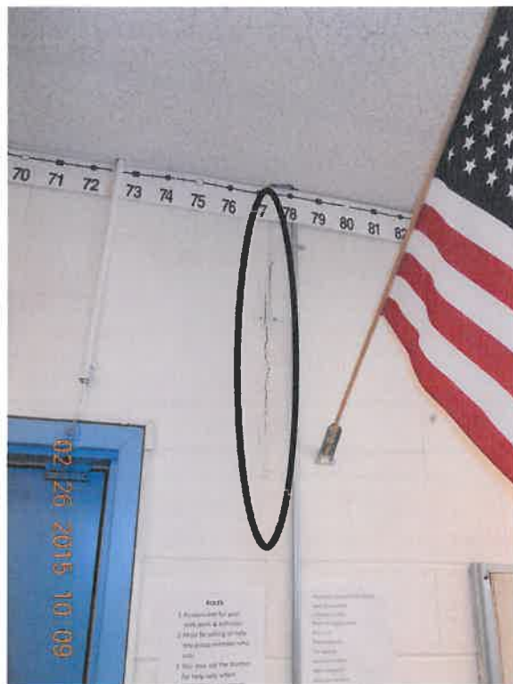
Room 7 - wall crack
