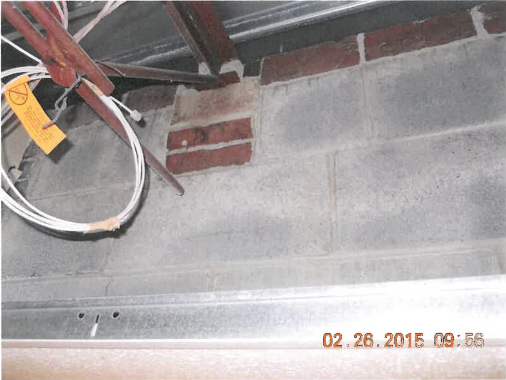
Room 5 - no structural roof damage
