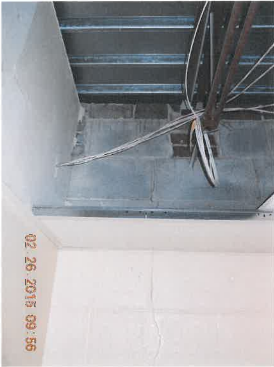
Room 5 - crack extends to point of support
